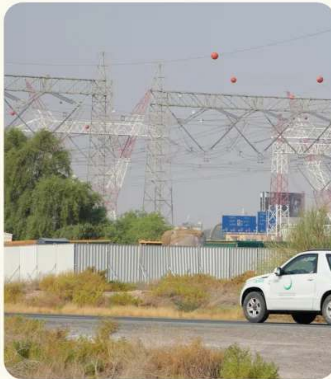
DEWA power facility
